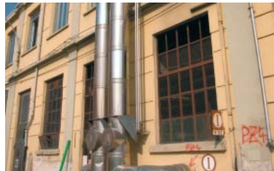
Aluminium pipes and office windows in the Pirelli building
